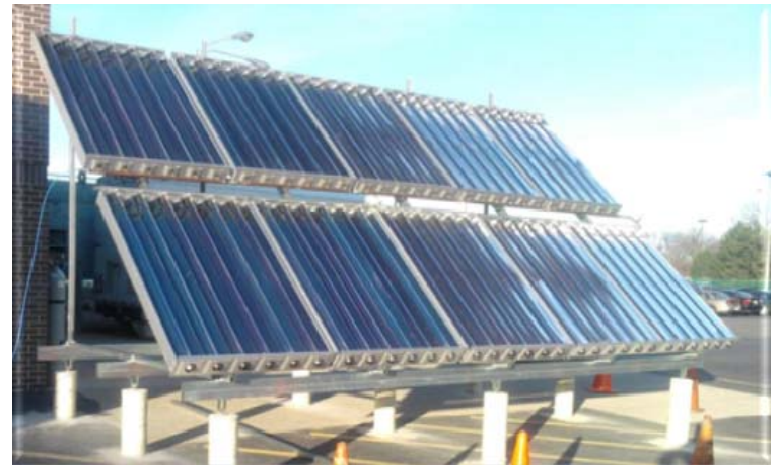
b2u Solar 10kW array at Gas Technology Institute
